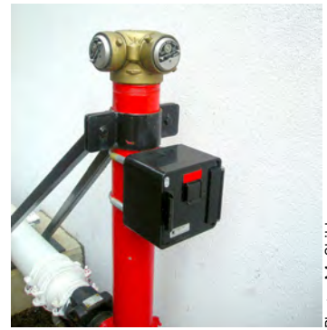
Figure 10.6. An FDC with locked plugs. The key is in the key box below the inlets.
