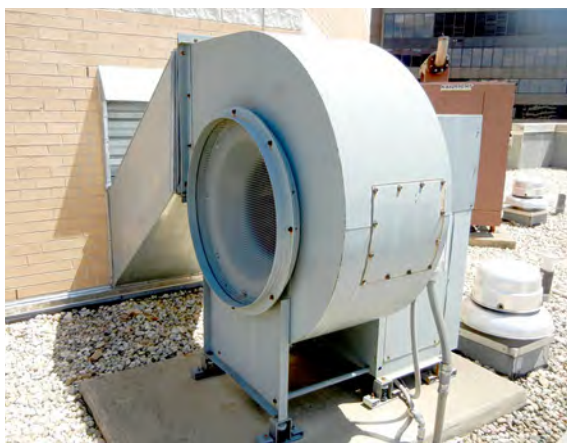
Figure 12.12. A stair pressurization fan.
