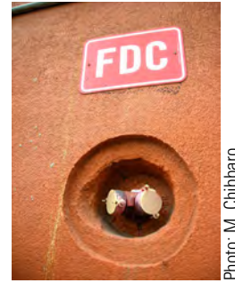
Figure 10.13. An FDC recessed into a wall. Note the notch on left prevents hose lines from kinking.
