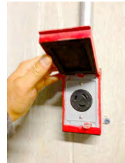
Figure 12.9. A weather-resistant outlet cover opened, showing a twist-lock type of outlet.
