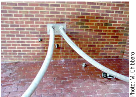
Figure 10.1. Charged hose lines connected to a wall-mounted FDC with two inlets.
