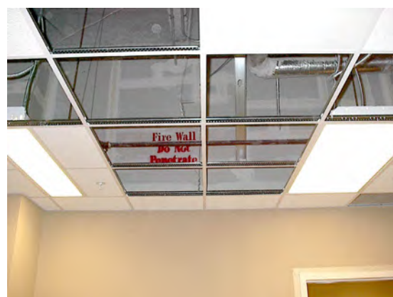
Figure 13.14. A “Do Not Penetrate” sign stenciled on a fire barrier wall above a suspended ceiling. The sign is intended to warn workers modifying the utilities located in the space above the ceiling.
