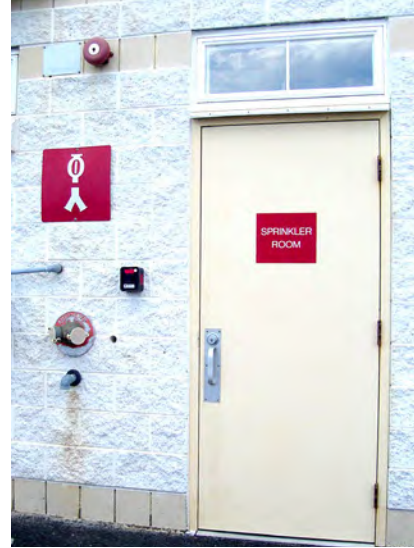
Figure 8.7. The sign on this door indicates that a sprinkler control valve is located within the room.
