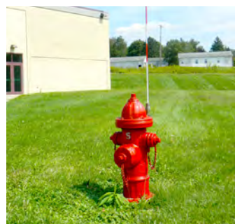
Figure 4.7. A dry barrel fire hydrant.
