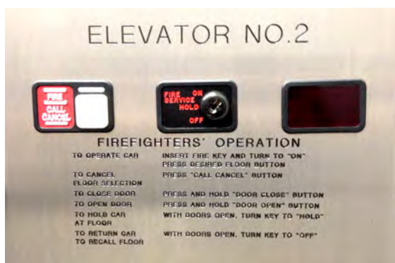
Figure 6.12. Elevator cab controls for Phase 2 firefighter operation.
