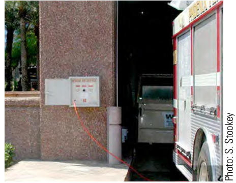
Figure 12.7. An exterior FDCP being supplied by a fire service mobile air unit.
