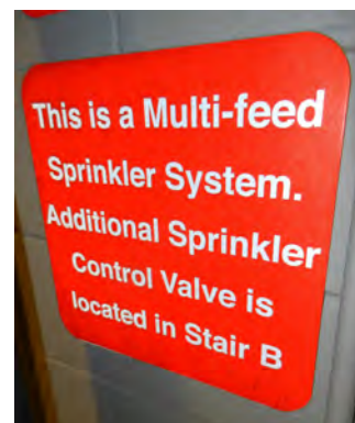
Figure 8.8. A sign near a sprinkler control valve indicating the location of the other valve that controls the same system.
