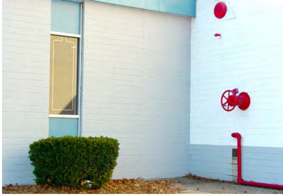
Figure 8.5. A wall control valve next to a window. Fire issuing from this window could prevent access to the valve.
