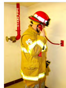
Figure 11.14. A firefighter training to use a handset in a remote jack located inside a stair.
