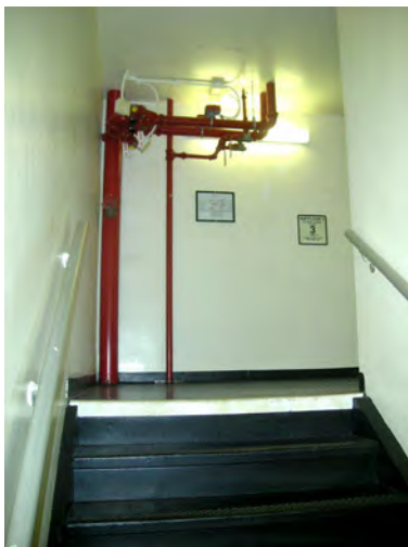
Figure 8.6. A sprinkler zone control valve in a stair enclosure.
