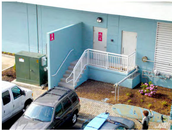
Figure 4.5. An outside door to a fire pump room identified by the red sign.
