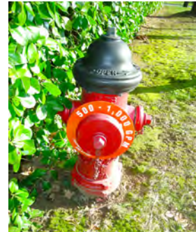
Figure 4.8. A fire hydrant with flow indicator sign.
