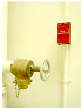
Figure 12.8. A firefighter emergency power outlet next to a standpipe fire hose connection.
