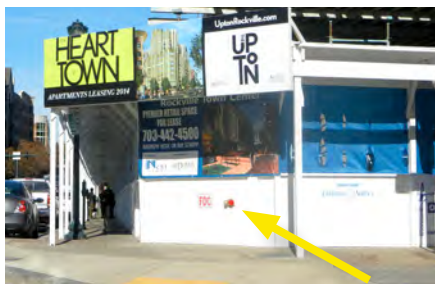
Figure 13.6. A temporary FDC (see arrow) feeding a standpipe being installed as this building rises.
