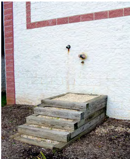
Figure 10.12. A platform built up to reach an FDC. This creates an unnecessary fall hazard.
